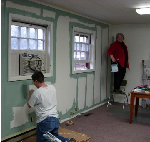
Painting a wall at an emergency shelter for victims of domestic violence. (January 2016)
